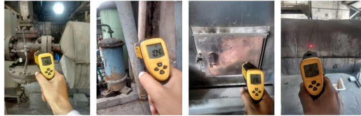
Figure 3. Surface temperature of steam distribution pipes in RTM plants at various locations
