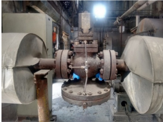
Figure 6. PRV installed in RTM plant for pressure reduction of steam
