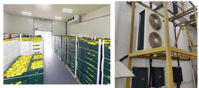
Figure 1. (A) Internal storage unit and (B) External unit of condenser used in setup
