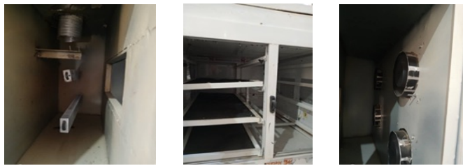
Figure 13. Resistance, drying chamber and fans
