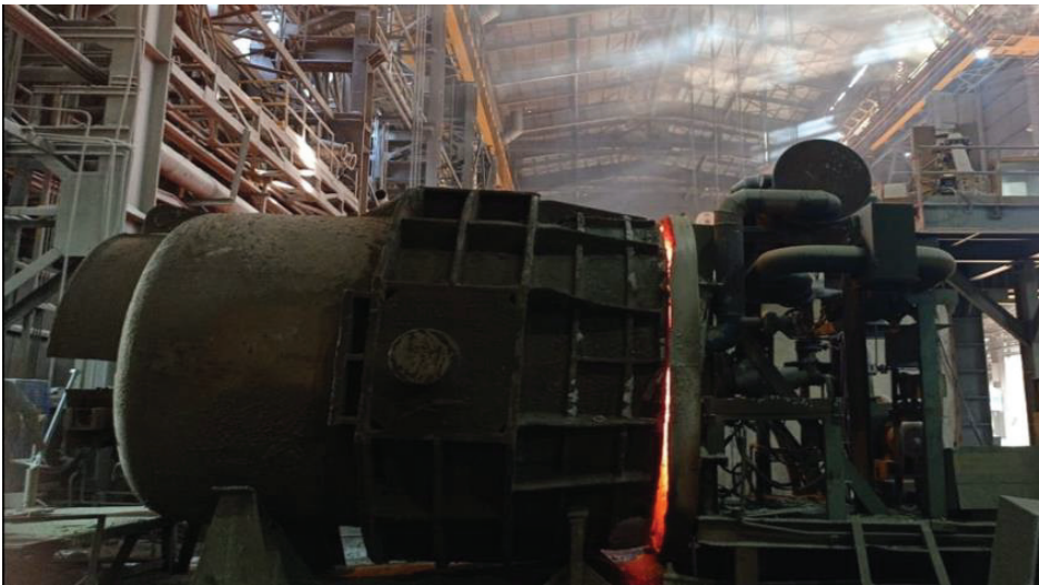
Figure 3. Illustration of the ladle preheating with a heat exchanger at JSW.
