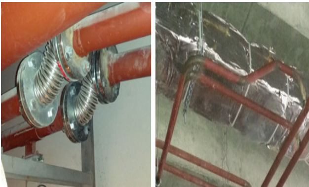
Figure 4. Application example of mechanical application fault (B1).
