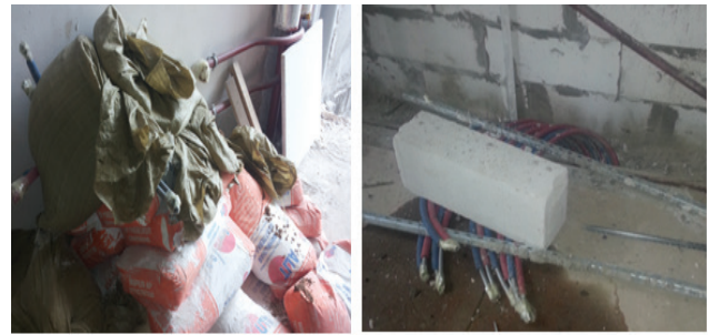
Figure 5. Application example of construction system fault (B3).
