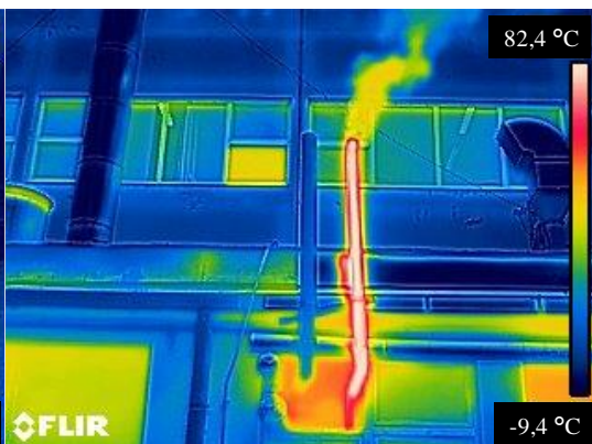
Figure 9. Thermal image of vented pipe and condensate flash losses
